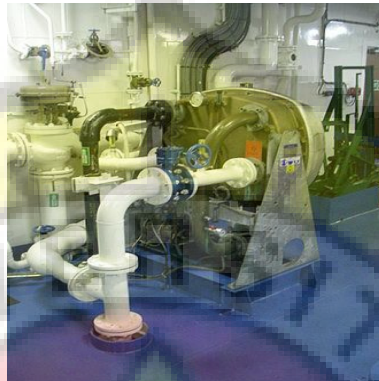
Gambar 2.1.1 Fresh Water Generator
