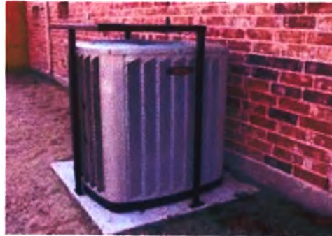
Gambar 2.13 Air Cooled Condenser
