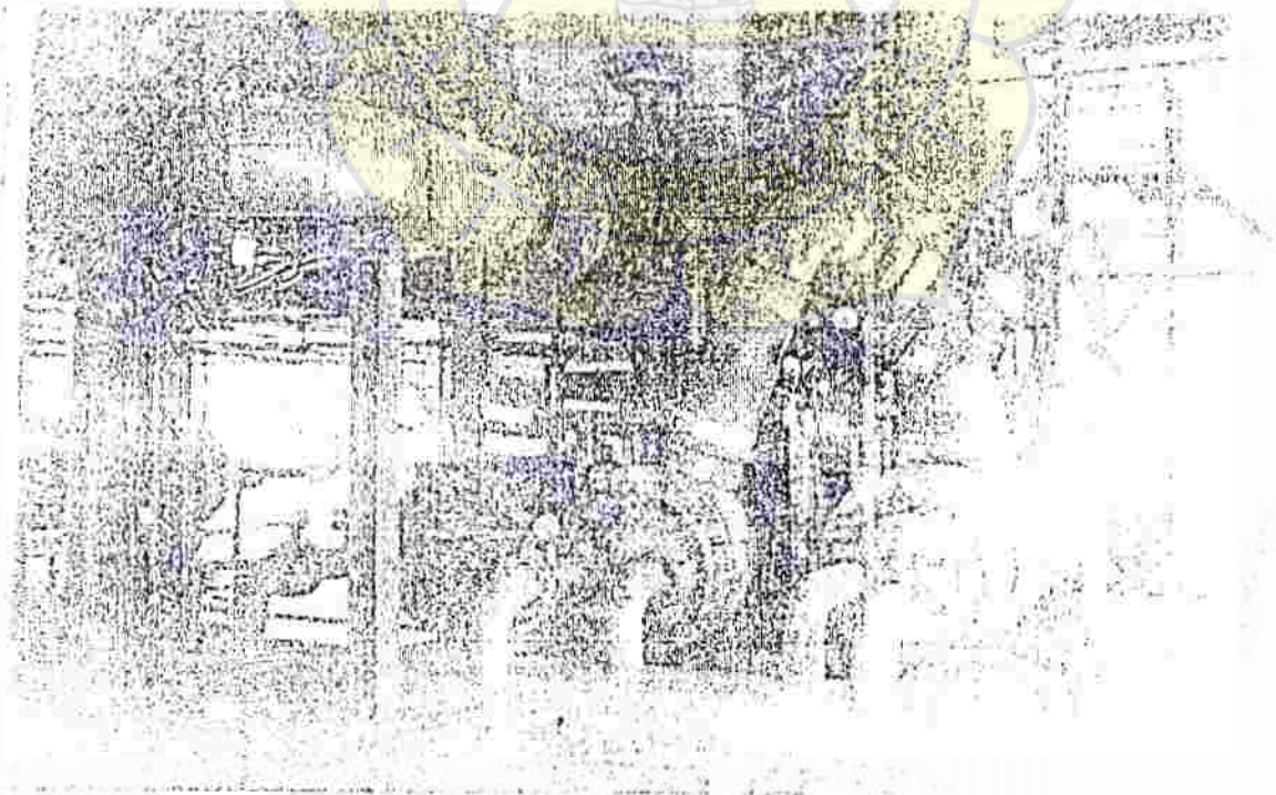
AIR COMPRESSOR CP-11
