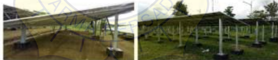
Gambar 2.1 PLTS Ground (Ditjen EBTKE, 2020)
