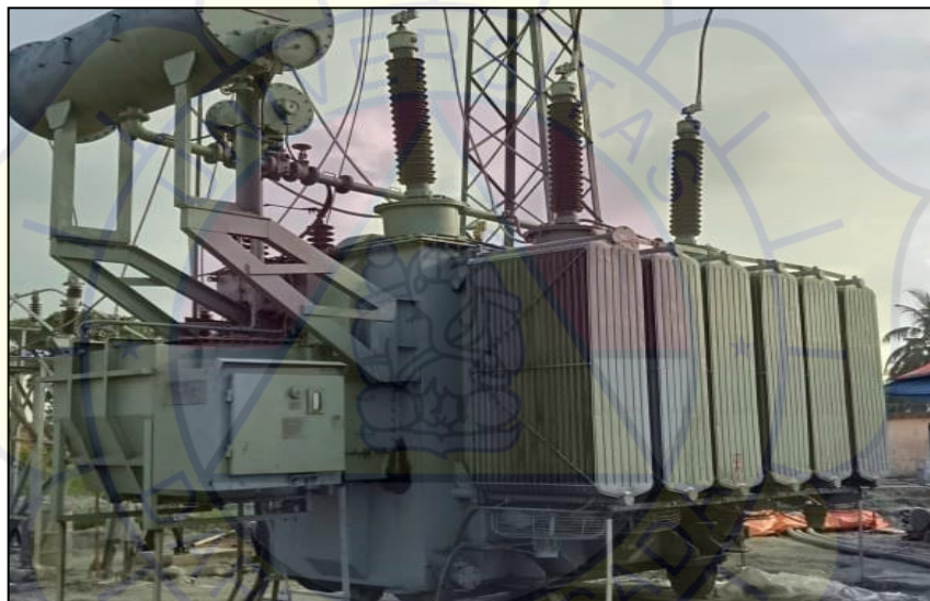
Gambar 2. 5 Unit Auxiliary Transformator
