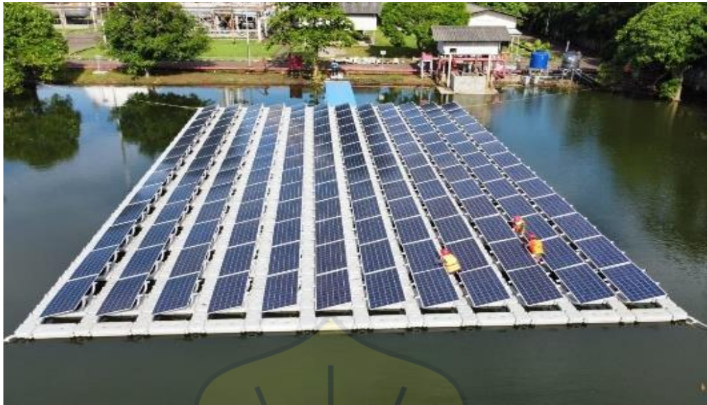
Gambar 2-5 PLTS Terapung/Floating Solar Panel
